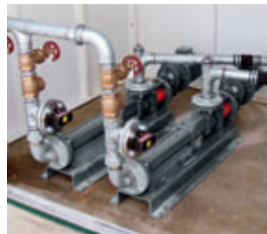
Waste water pumping
